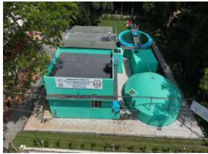
360 KLD STP at General Hospital, Thrissur
