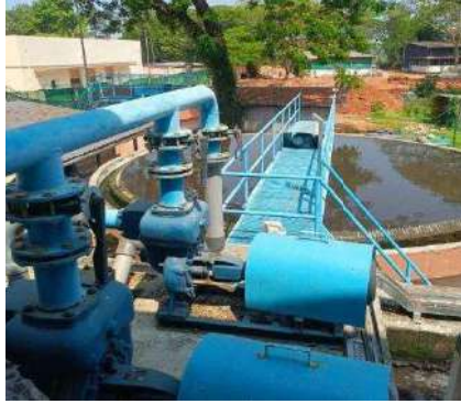
500 KLD STP at Kozhikode medical College
