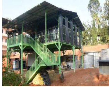
1 MLD STP at Kozhikode medical College
